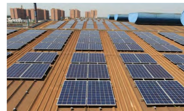
PV power generation system
