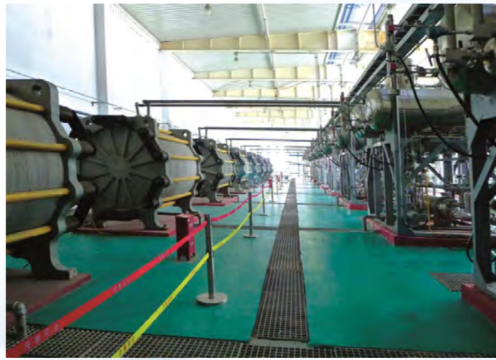
Super-large water electrolytic hydrogen generator of CSSC No. 718 Research Institute
